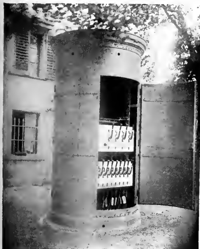
FIG. 5.—SECONDARY SIDE OF TRANSFORMER HOUSE.
